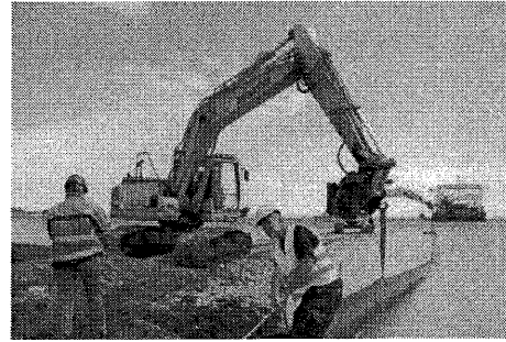
Construction of offshore substation platforms and transmission cables to deliver power onshore to the existing power grid. (Photo: Energinet.dk).
