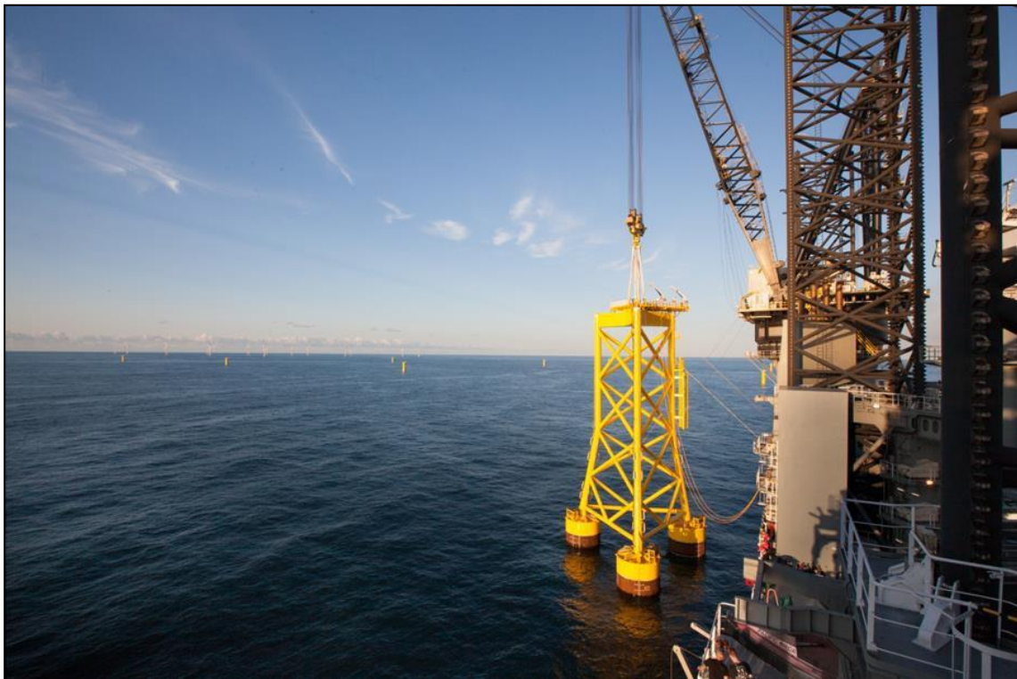
Figure 3-6 Example of possible foundations for the wind power plant: the suction bucket foundation (Image: Borkum Riffgund).
